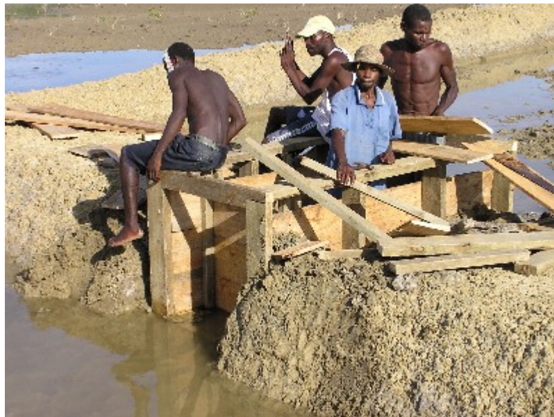
Construction of a secondary gate in Mkadam site in Tanzania with the assistance of former volunteer Edwin Requentina
