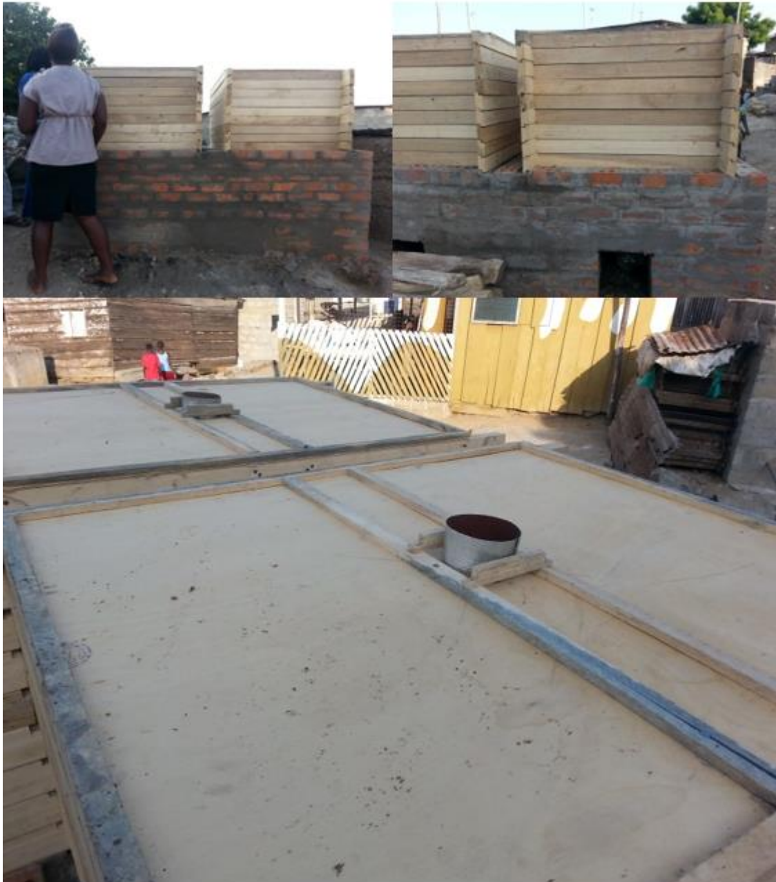
Figure 2. A finished constructed Morison Oven for fish processors in Winneba in the Central Region of Ghana.
