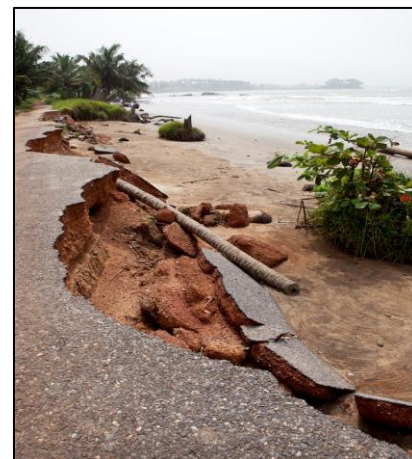
Figure 2: Washed feeder road along Ankobra beach
