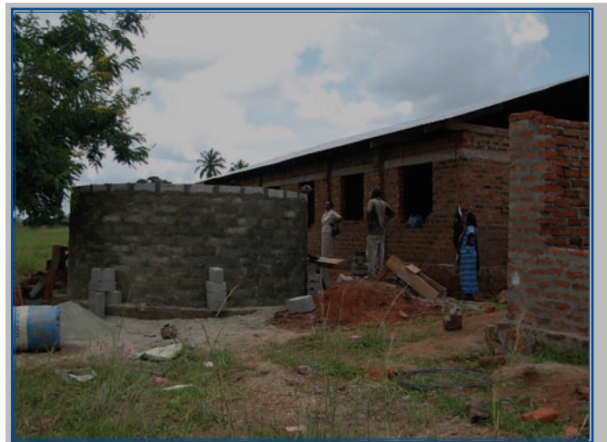
Constructing water tanks for schools in Tanzania's Wawi Watershed is critical to address current climate issues and to improve for health and sanitation of the community.
